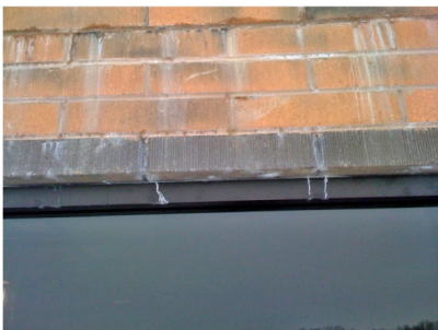
Mortar or masonry run-off onto anodized window frame
