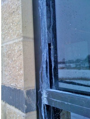
Mortar run-off onto anodized window frame
