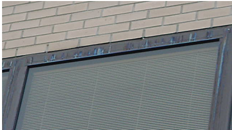
Damage to anodized framing from mortar and brick wash
